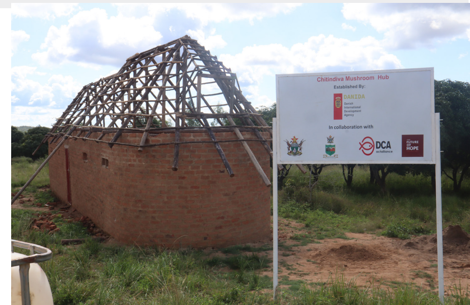
Chitindiva Mushroom Hub located at Chitindiva Primary School during construction. It is one of three mushroom hubs constructed by the Utariri Pilot Project in Hurungwe
